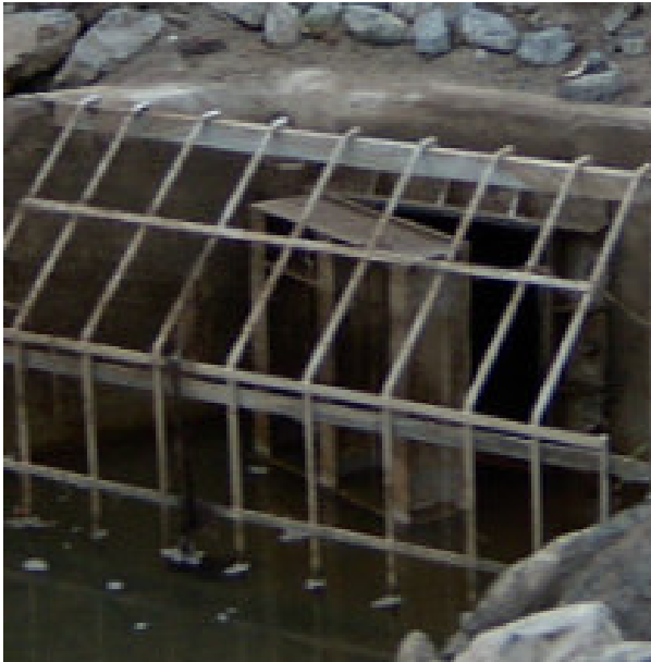
Photo 3 - Side Opening Flap Gate at Nanaimo BC
