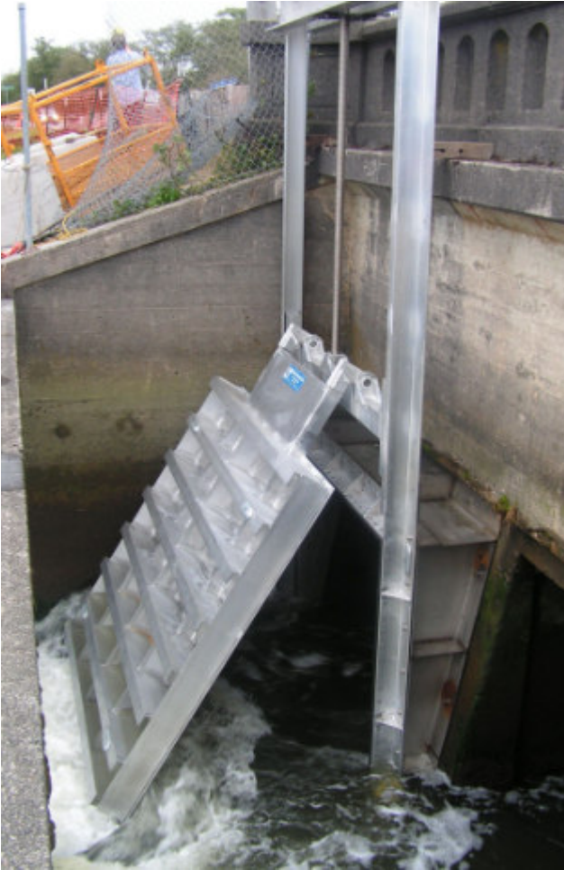
Photo 4 - Combination Gates were installed to replace existing timber flap gates on Highway 101 Bridge crossing Chinook River.
